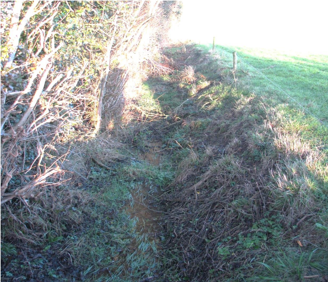
Figure 12-9: Intermittent drainage ditch which is dry in summer but flowing in winter (Photo: Donal Daly).
