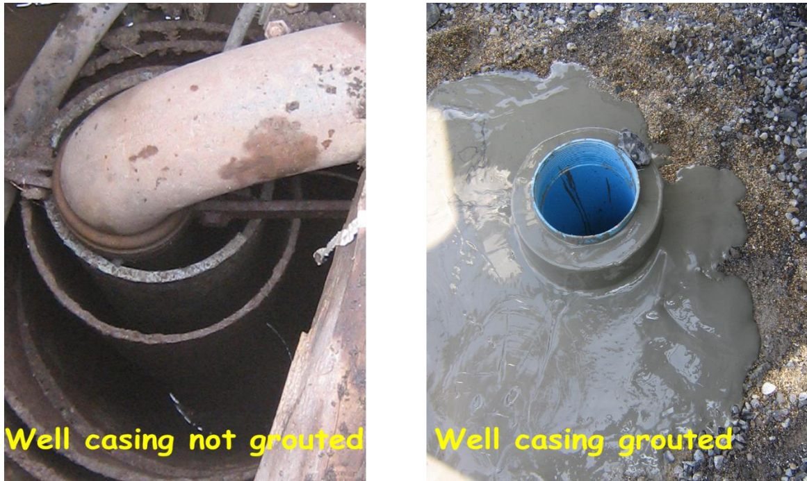
Figure 13-6: Water containing pollutants can readily flow down the outside of the casing if not grouted properly (Photos: David Ball).
