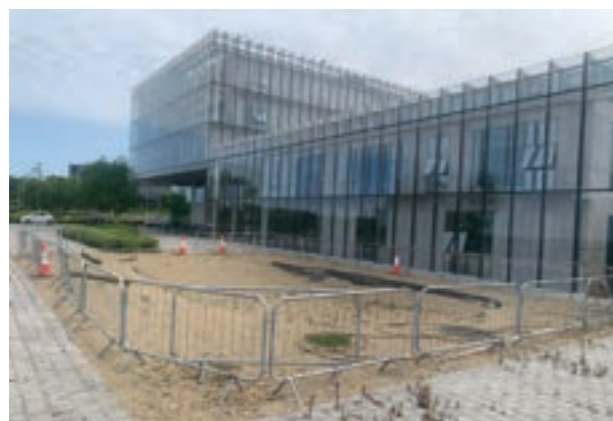
Figure 22: Collapsed Attenuation Tank - Wexford County Council
